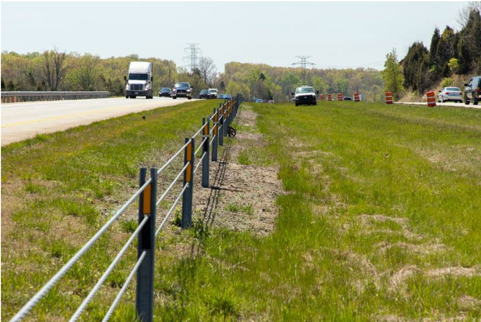
Figure 8: View of Plots in the Cable Barrier Trial on April 26, 2021 (328 Days After Treatment) Spray pattern on both sides of the cable barrier, and how well some treatments are still suppressing vegetation.
