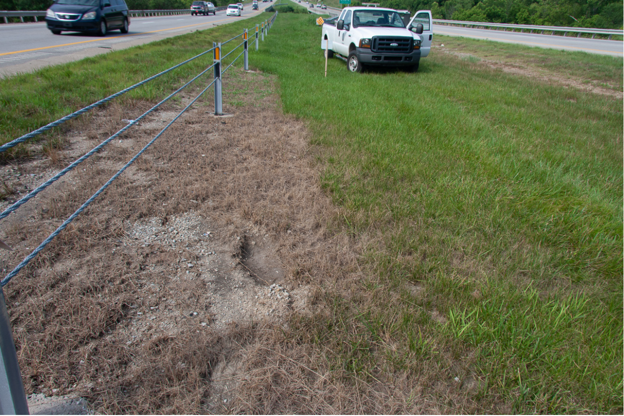
Figure 3: View of Treatment 2 and 1 plots the Cable Barrier Trial on July 3, 2018 (41 Days After Treatment) Treatment 2 (Roundup ProMax + Sahara) was sprayed on the plot in the foreground. Note the turf damage beyond the initial spray pattern as seen on the plot closer to the truck which only had Roundup ProMax applied.
